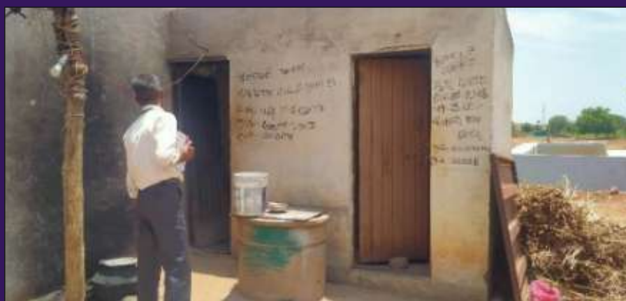
Antaragange village Medakinal GP Raichur Toilets not in use, it is observed that the toilets are constructed but are used for storage and other purposes
